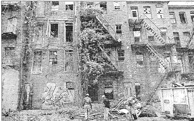
A demolition crew removes trash along the back side of 588-612 E. Main St. in Bridgeport on Tuesday. Plans are to save the dilapidated structure and create housing and retail space.
